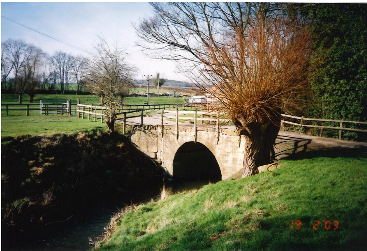
Bridge over the River Isbourne, looking west, 2003 (between points B and C)
